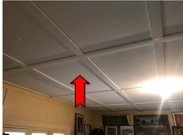
Photo 2. Interior, ground level, club room ceiling – assumed asbestos-containing fibre cement sheeting.
