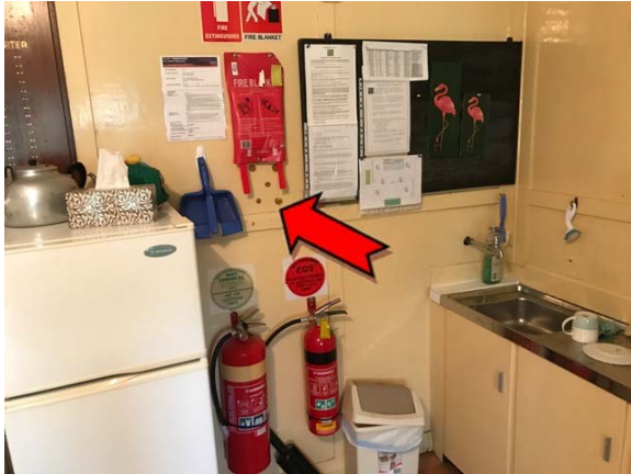
Photo 1. Interior, ground level, club room wall – asbestos-containing fibre cement sheeting.
